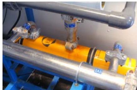
Energy Recovery Device
