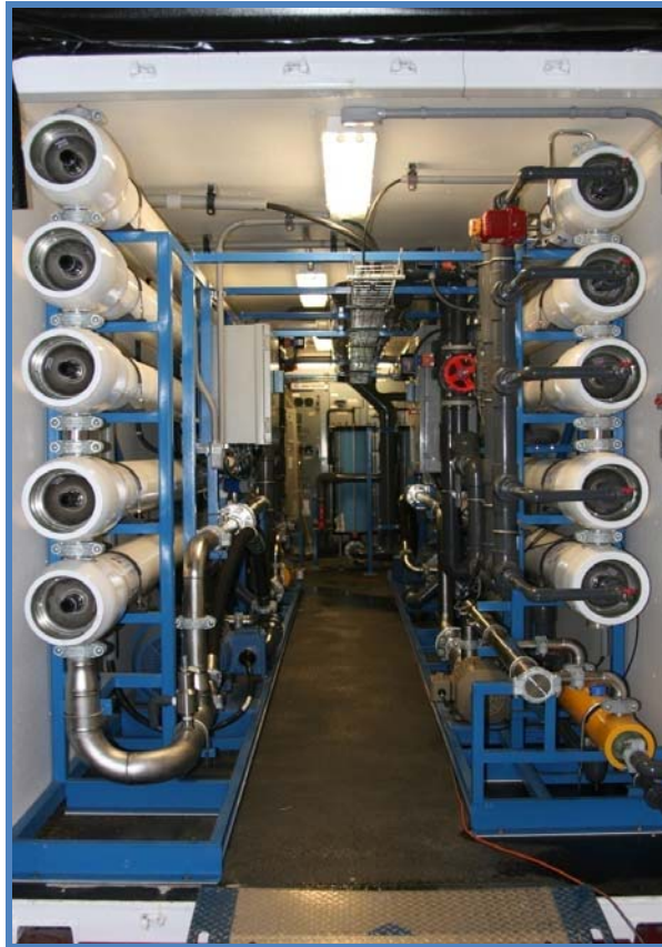
Figure 3: Photograph of Seven Seas Water SWRO 250,000 GPD Containerized Unit
